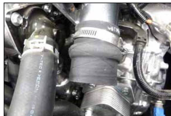
16. Install the provided step coupler onto the upper charge tube but do not secure.
